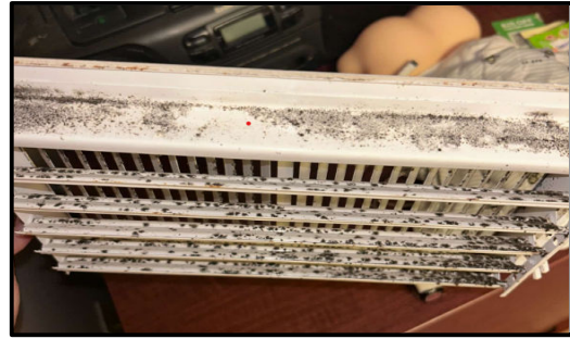
Mold in Air Vent Fanning – Room #201
