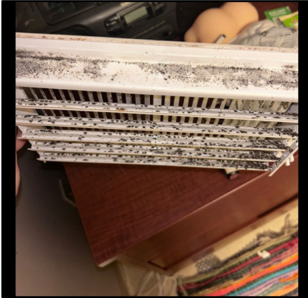
Natalie Hough Mold Covering Air Vent Fanning Hall – Room #201-1 Photo Taken: 9/16/2025
