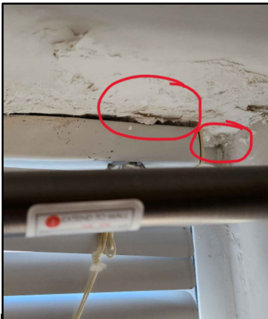
Johannah Maurer Damaged Ceiling from Excessive Condensation Johnson Hall – Room #470 Photo Taken: 11/15/2025
