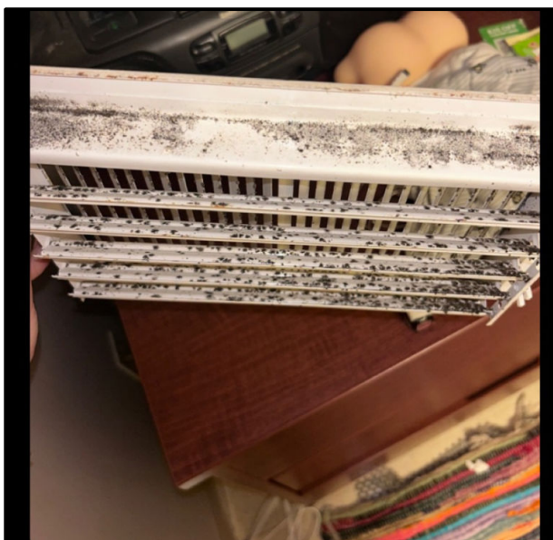
Natalie Hough Mold Covering Air Vent Fanning Hall – Room #201-1 Photo Taken: 9/16/2025
