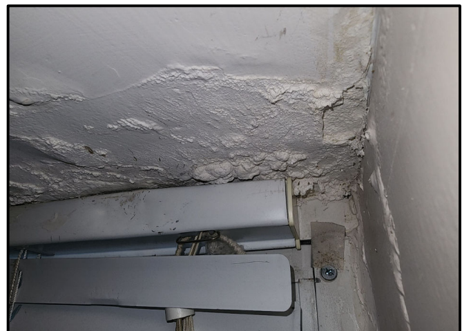
Johannah Maurer Damaged Ceiling from Excessive Condensation Johnson Hall – Room #470 Photo Taken: 11/15/2025
