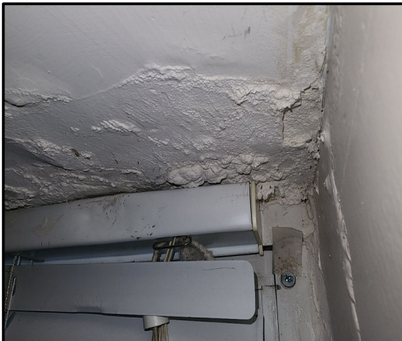
Johannah Maurer Damaged Wall & Ceiling from Excessive Condensation Johnson Hall – Room #470 Photo Taken: 11/15/2025
