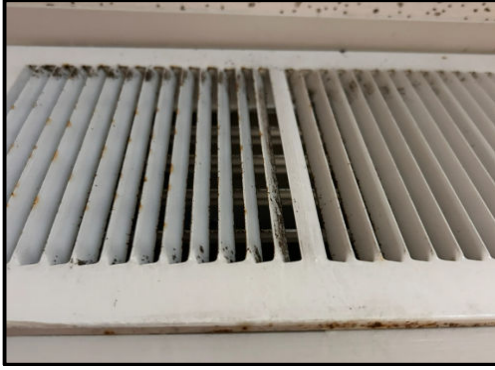
Rust and Mold Growth in Air Vent Fanning – Room #108
