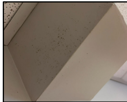
Mold Growth on Wall Fanning – Room #108
